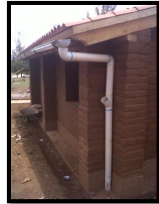
Figure 7. Rainwater catchment system
